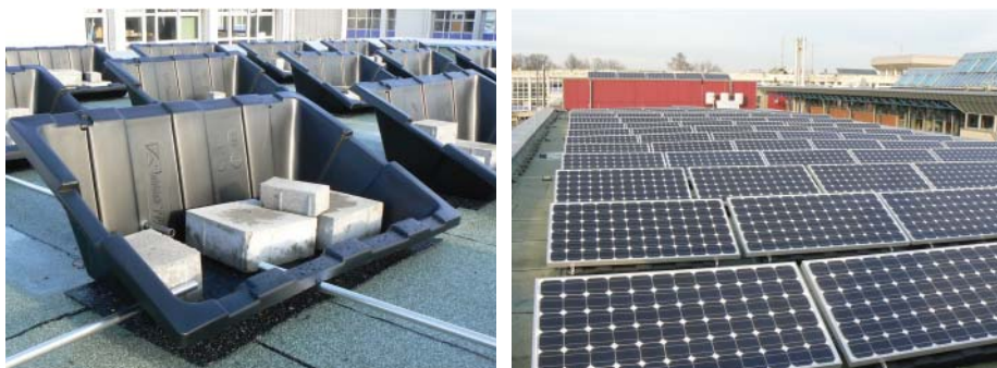
Figure 6.31 Flat-roof system on the roof of Münster University of Applied Sciences in 2008: The modules are placed in plastic tubs that are weighed down by paving stones.
