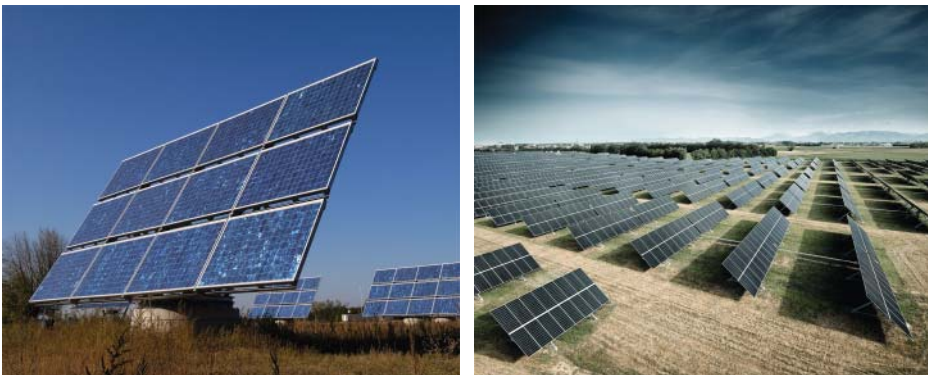
Figure 6.29 Tracked ground-mounted plants: Dual-axis Solon-Mover and a single-axis system with horizontal axis. Source: © SOLON Energy GmbH, Urnato/© SOLON.
