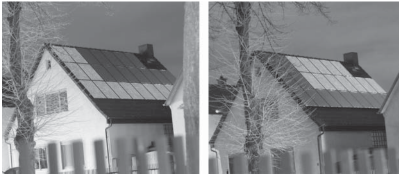
Figure 9.19 On-site examination of an on-roof plant: Subsequently string 1 and string 2 are energized to inspect the modules for damage. Photos: M. Diehl.
