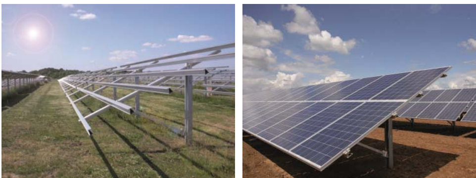
Figure 6.27 Typical construction of a ground-mounted plant: Galvanized steel posts are rammed into the ground and serve as the base for the module panel support. Source: Schletter GmbH.
