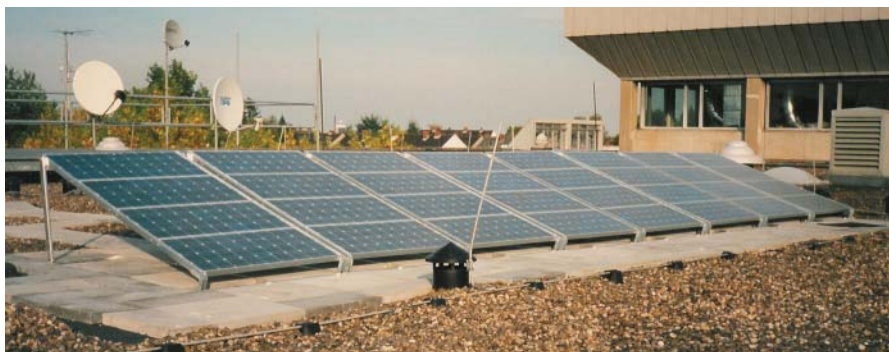
Figure 6.30 Photovoltaic plant at Münster University of Applied Sciences from 1994: The aluminum support structure is held down by means of flagstones. Source: W. Göbel.
